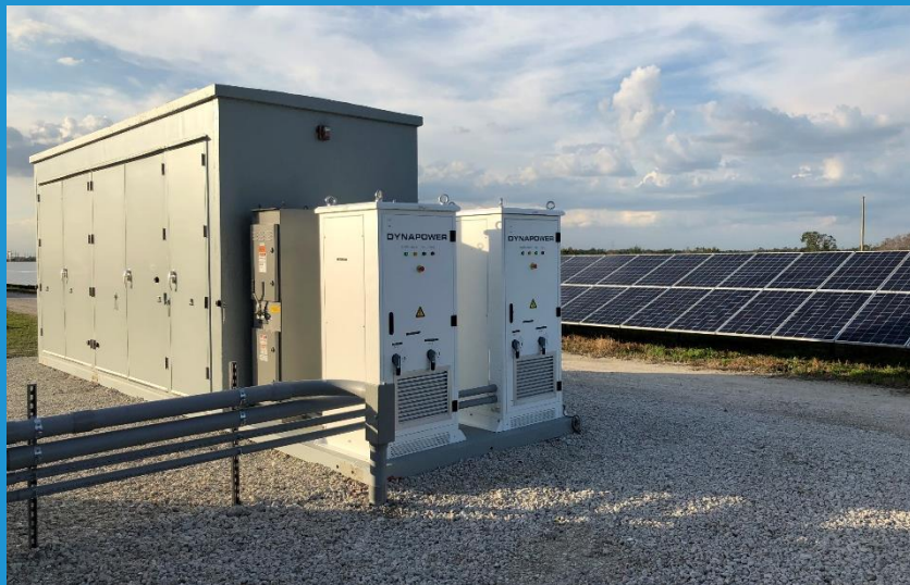
Battery Storage at FPL Citrus Solar Energy Center
