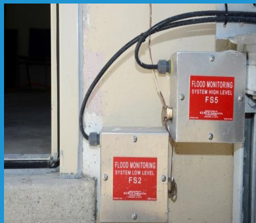
Substation Flood Monitor
